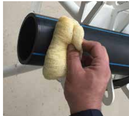
3-Clean pipe scraped area . Note: do not touch the scraped area with bare hands after scraping and cleaning.
